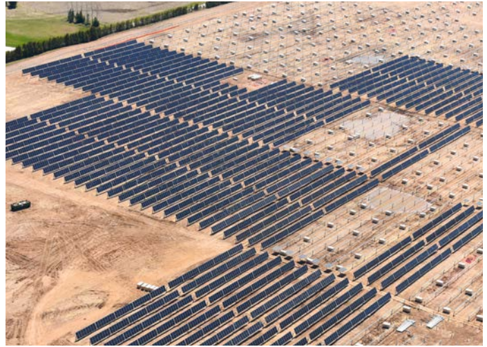
Solar panels installed on a joint Wisconsin Public Service and Madison Gas and Electric large-scale solar project in Two Creeks, Wisconsin.
