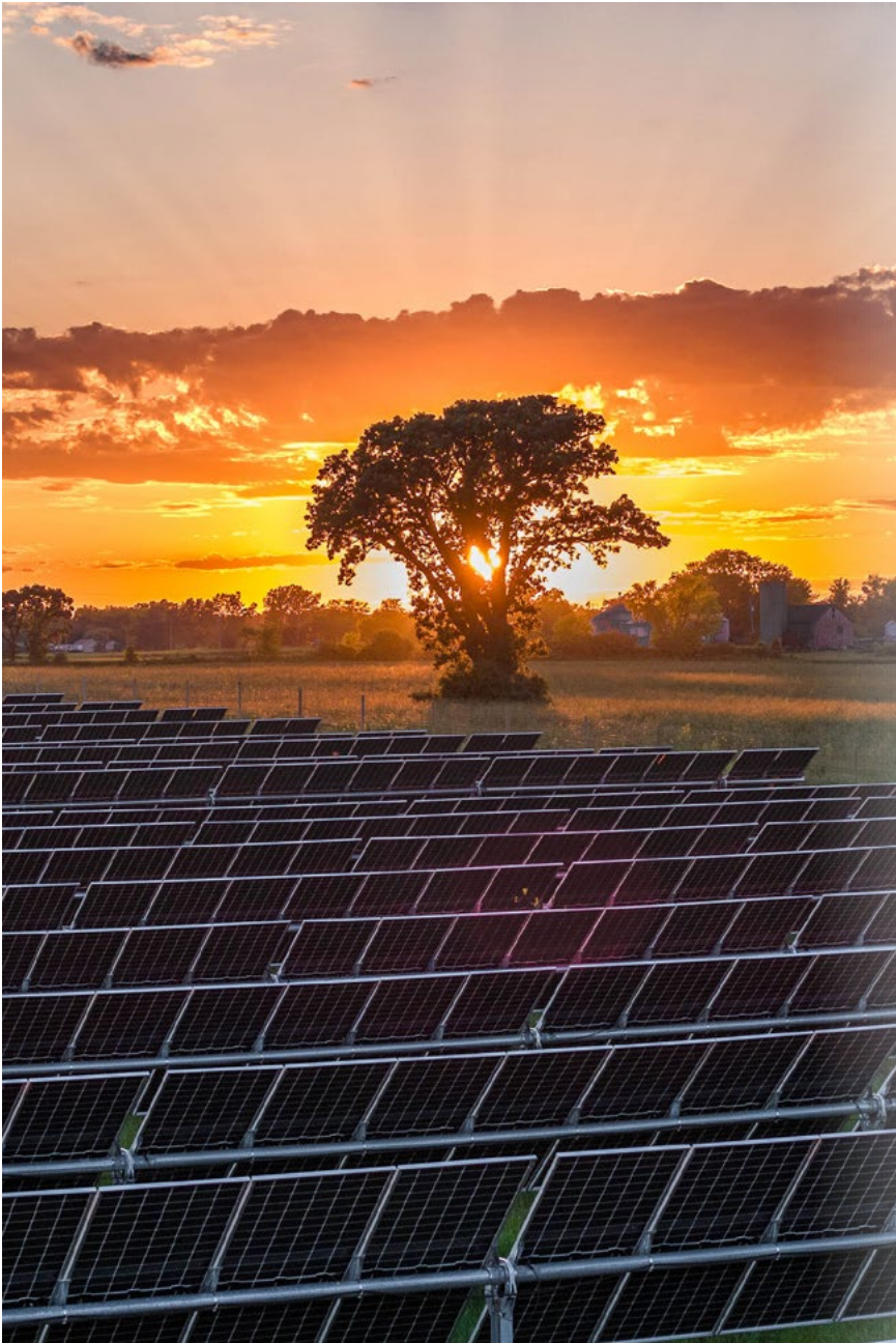
Paris Solar-Battery Park, Paris, Wisconsin
